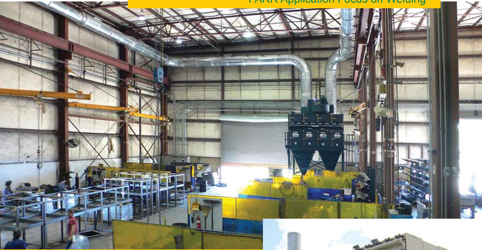
GS48 with Integral HEPA Filters on Weld Fumes
